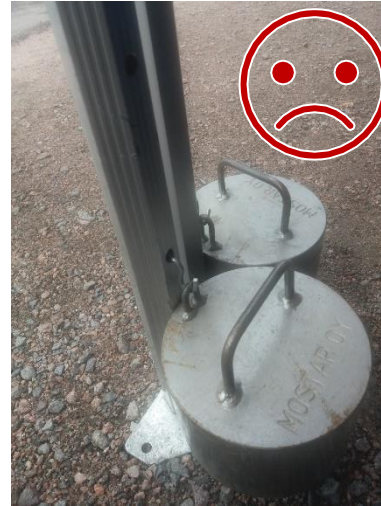
The steel hook is unlocked. Steel will cut aluminium, making the fastening ineffective.
