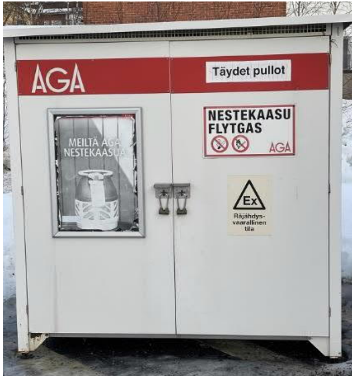
Image 2. A gas cylinder cabinet with a lock and all necessary labels.
