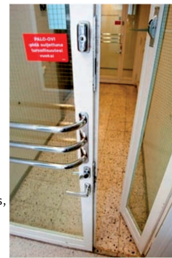
An open fire door is of no use in case of a fire.
